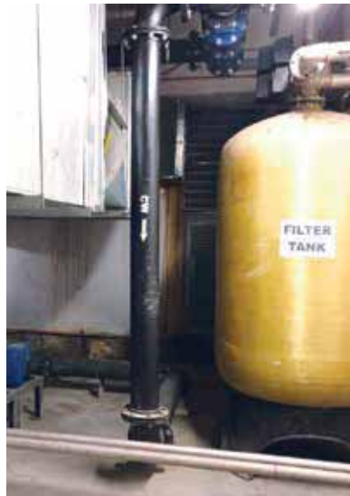
(Image 4: Level 1 Water Storage & Filtration Tank)
