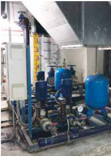
(Image 3: Level 1 Pump Room & Water Storage)
