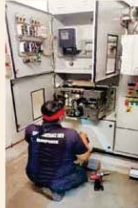
Figure 18: Major service and maintenance work of high tension and low voltage electrical panel at the building
