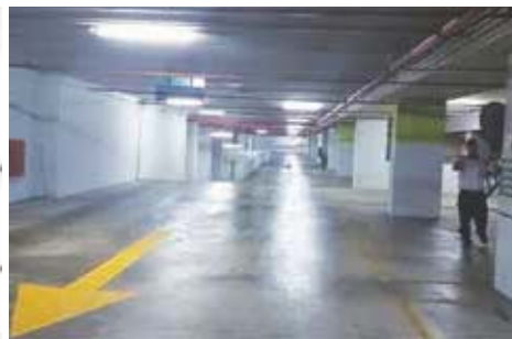
Figure 28: Installed energy efficient LED lighting
