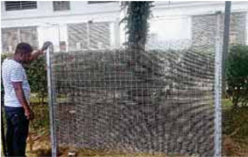
Figure 17: Installation of perimeter anti-climb fencing at Quill Building 1 (DHL 1) & Quill Building 4 (DHL2)
