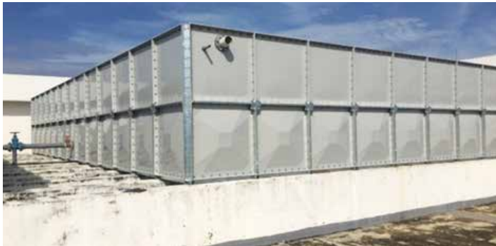
Figure 15: Sentral Building 4 – Finished installation works of new FRP Water Tank for HSE initiative
